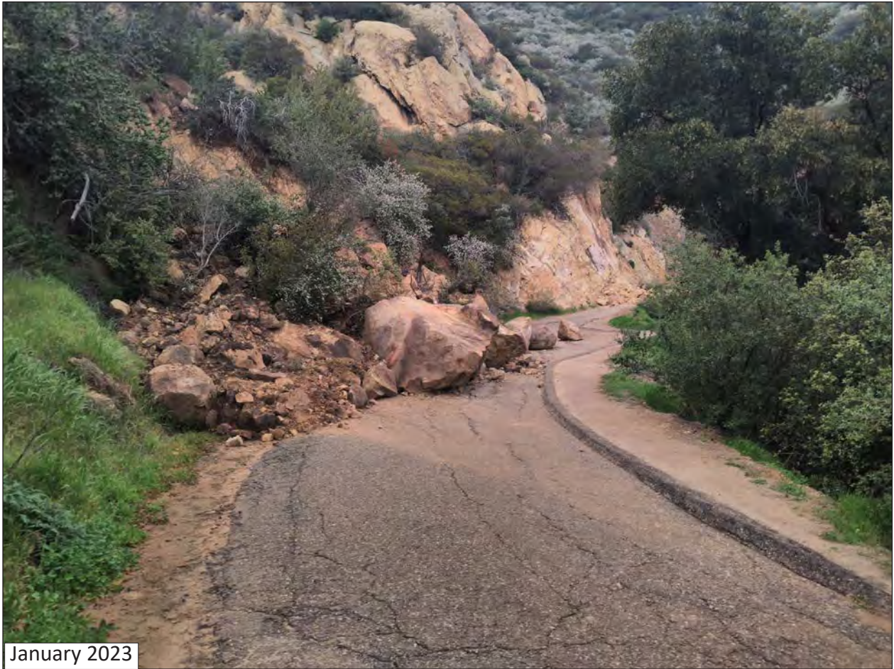
Photograph 3. Spyglass Ridge Road Area 1 with slope failure, looking north.
