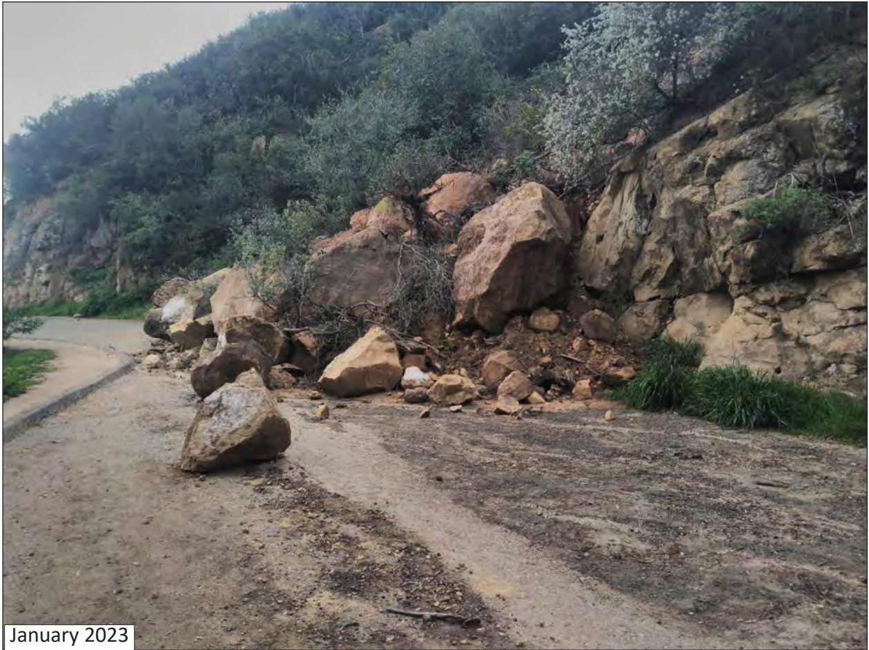
Photograph 5. Spyglass Ridge Road Area 2 with slope failure, looking south.
